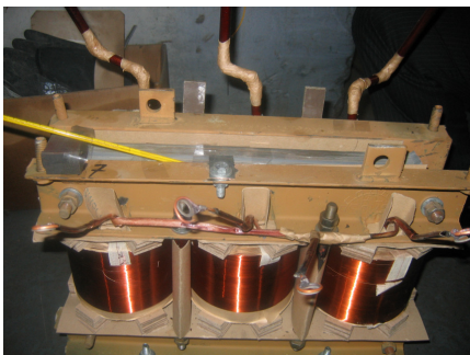
Inside view of transformer with CSIO fabricated FBG mounted
