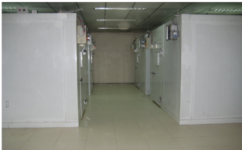
Potato Storage chambers with sensors and electronic controls
