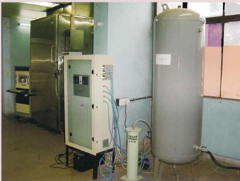
Controlled Atmosphere Storage System
