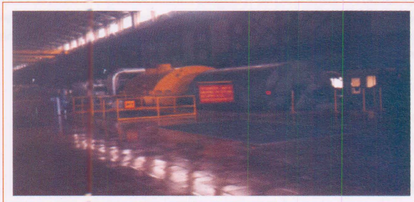
Site view of installation in Thermal Plant
